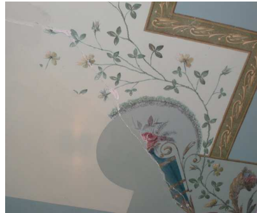
Cracked plaster in the dining room at the Vaile Mansion.
